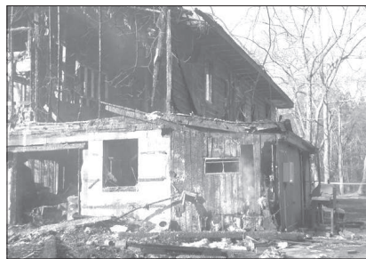
This home that housed 9 Hampden Sydney College athletes was completely destroyed by a fire last week. The fire also injured two residents, with one suffering serious burn injuries and having to be flown to VCU Medical Center.
